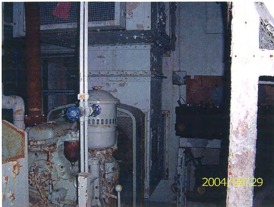
Photo 50 Genset - Module Train
