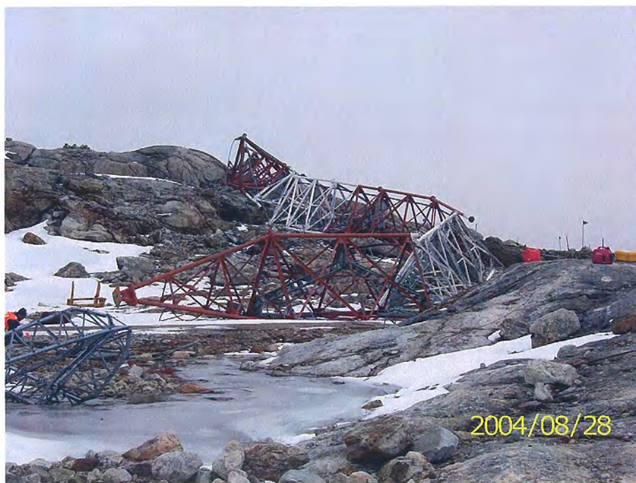
Photo 47 Downed antenna structure
