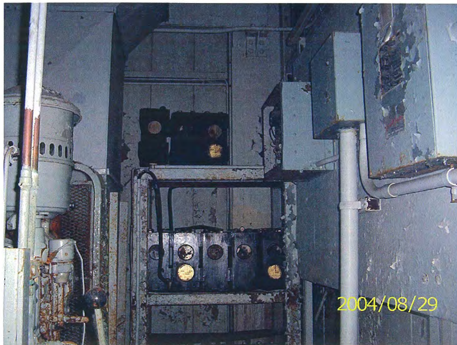
Photo 54 Batteries in Generator Room - Garage
