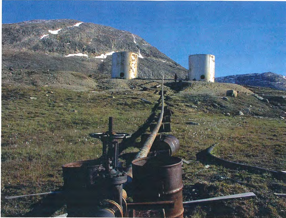
Photo 1 Beach Area POL tanks and pipeline, looking south
