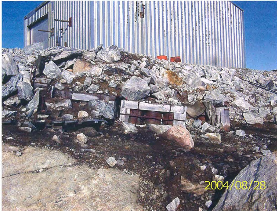
Photo 31 Staining below southwest corner of Garage
