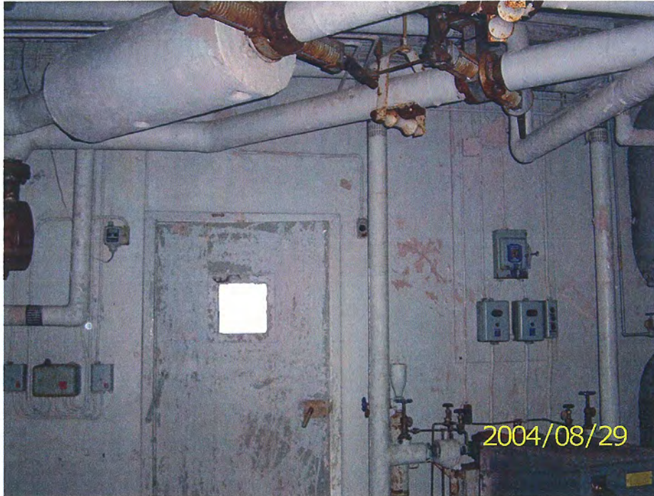
Photo 51 Typical piping in Warehouse
