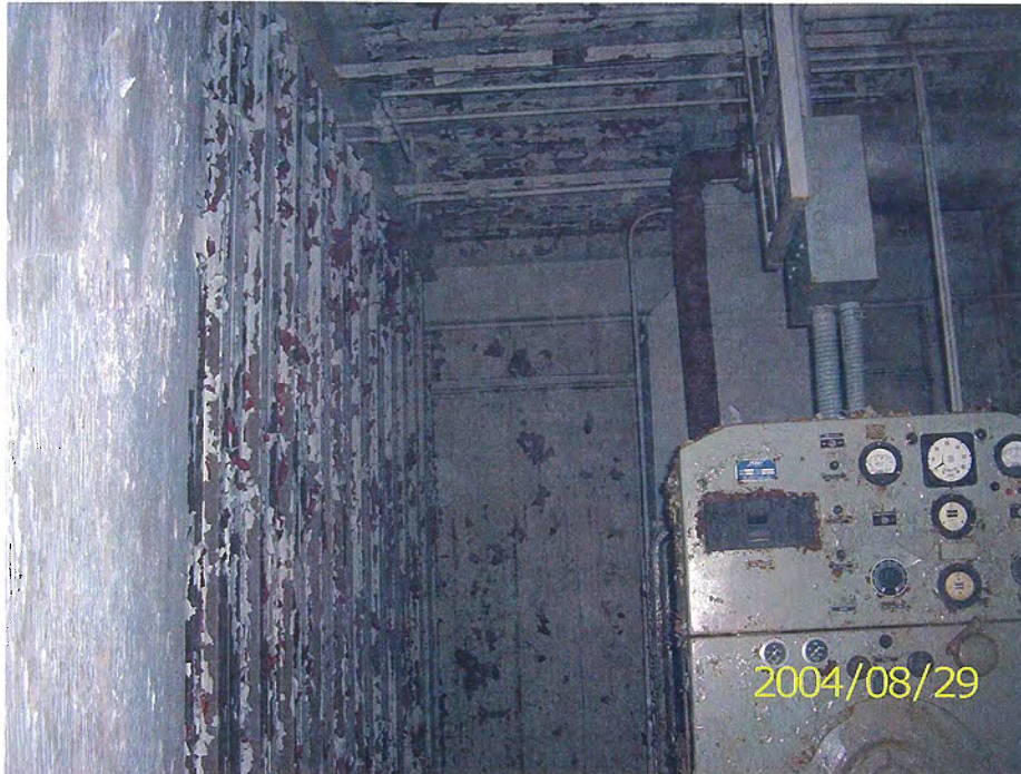
Photo 53 Genset and peeling paint in Generator Room – Garage
